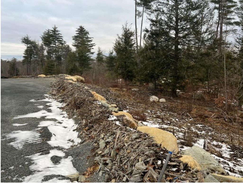
Northern edge of disturbance
